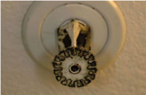
Corroded sprinkler head
